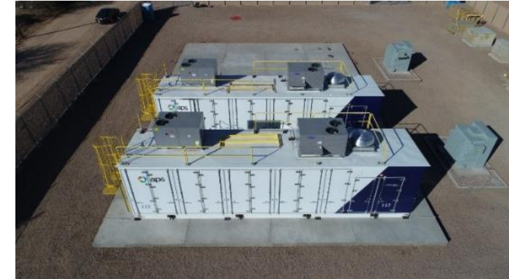
BESS at Punkin Center
